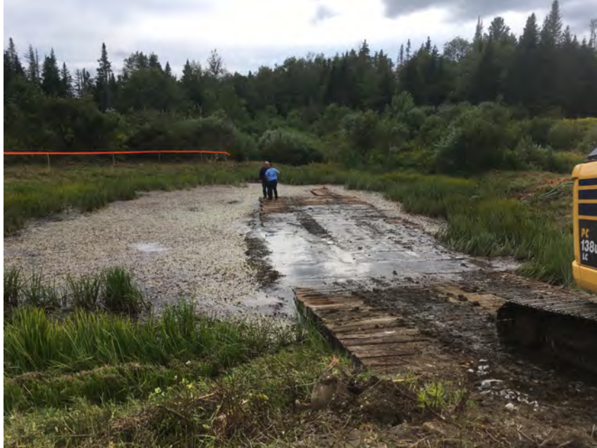
Beginning the dredging and repair of the snowmaking pond by Barkus Excavating (Readsboro, Vermont) in August 2019. View to southwest from parking lot.
