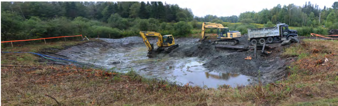
Bank repair and dredging nearly done, September, 2019. Maximum depth 7 ft. Planned capacity 300,000 gallons. View to west-southwest
